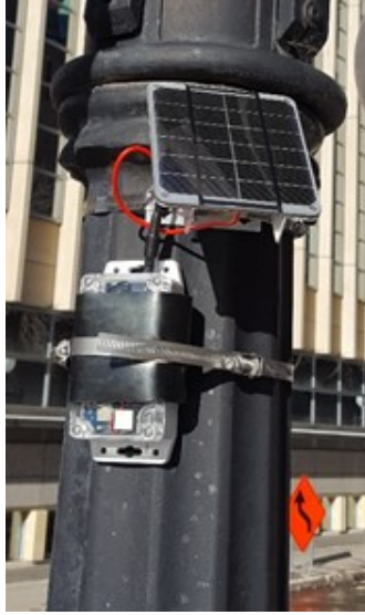
Figure 2.3 Solar-powered BLE on a street light post.
