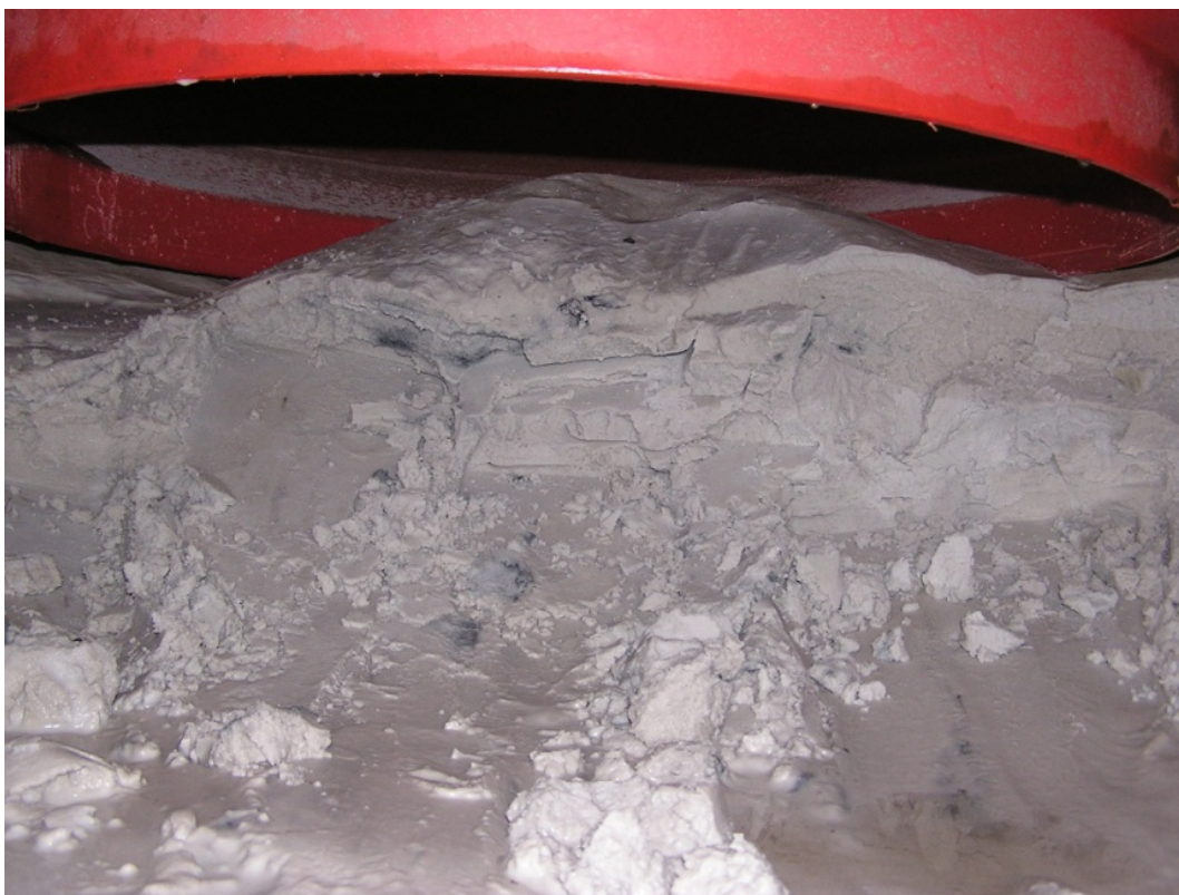
Figure 3-7: Sediment cone near Downstream Defender benching skirt
