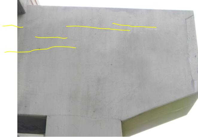
Figure 10.2. Cracking along straddle bent
