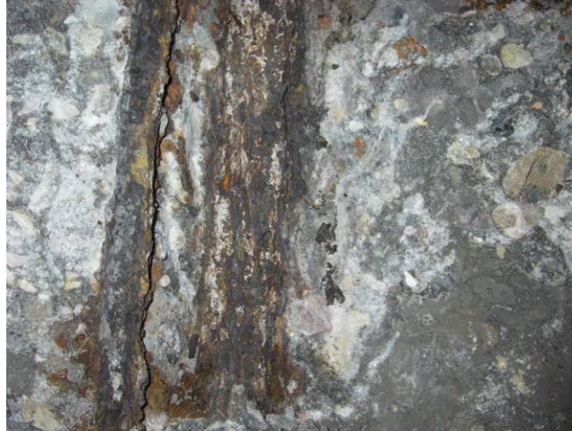
Figure 6.32. Corrosion on tendon B28
