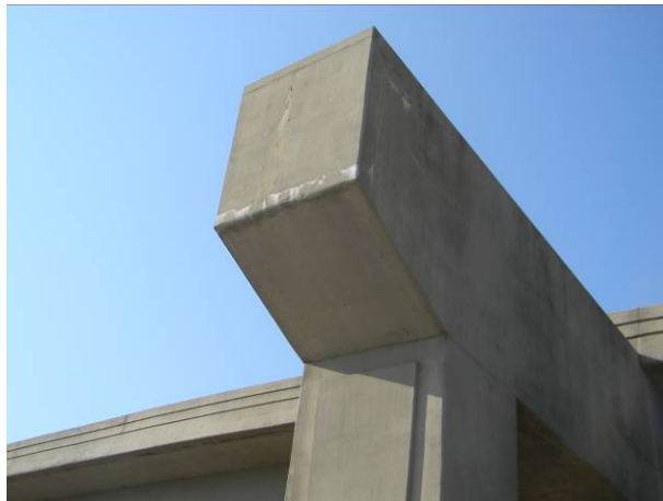
Figure 10.1. Pier with cracking and efflorescence
