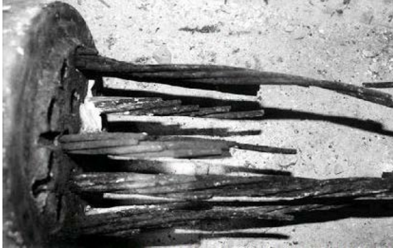
Figure 2.2. Strands corroded at anchor (Corven Engineering, 2002)
