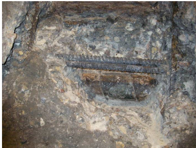
Figure 6.24. Shows tendon 16 with corroded duct
