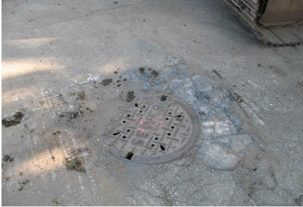
Figure 3.45. Rapid Patch manhole repair: Condition on August 26, 2015.
