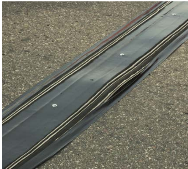
Figure 6: Wrinkles can cause vibrations and false axle signals
