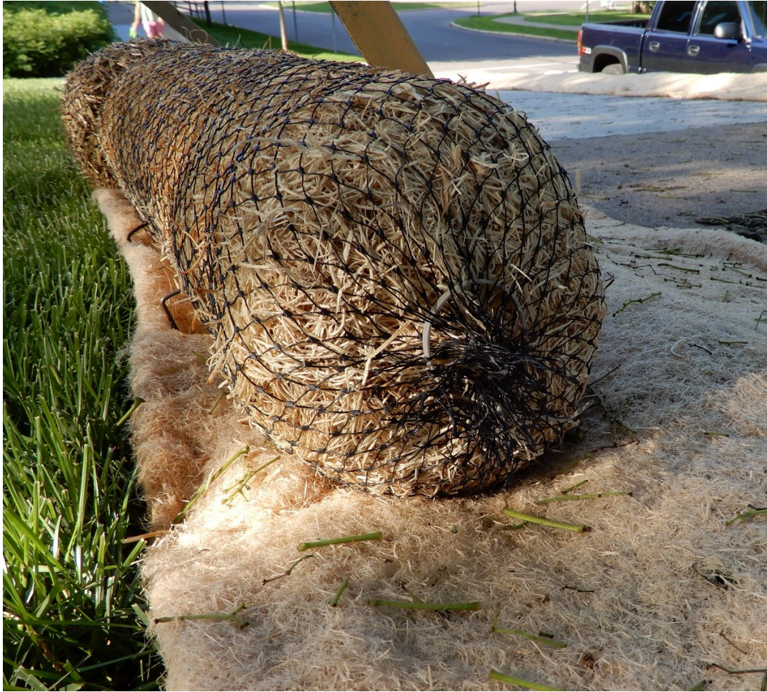
Figure 35 Sediment Control log installed using a wood fiber blanket foundation and staples placed at the leading edge. Traditional angled wood stakes are also placed along the downstream edge.
