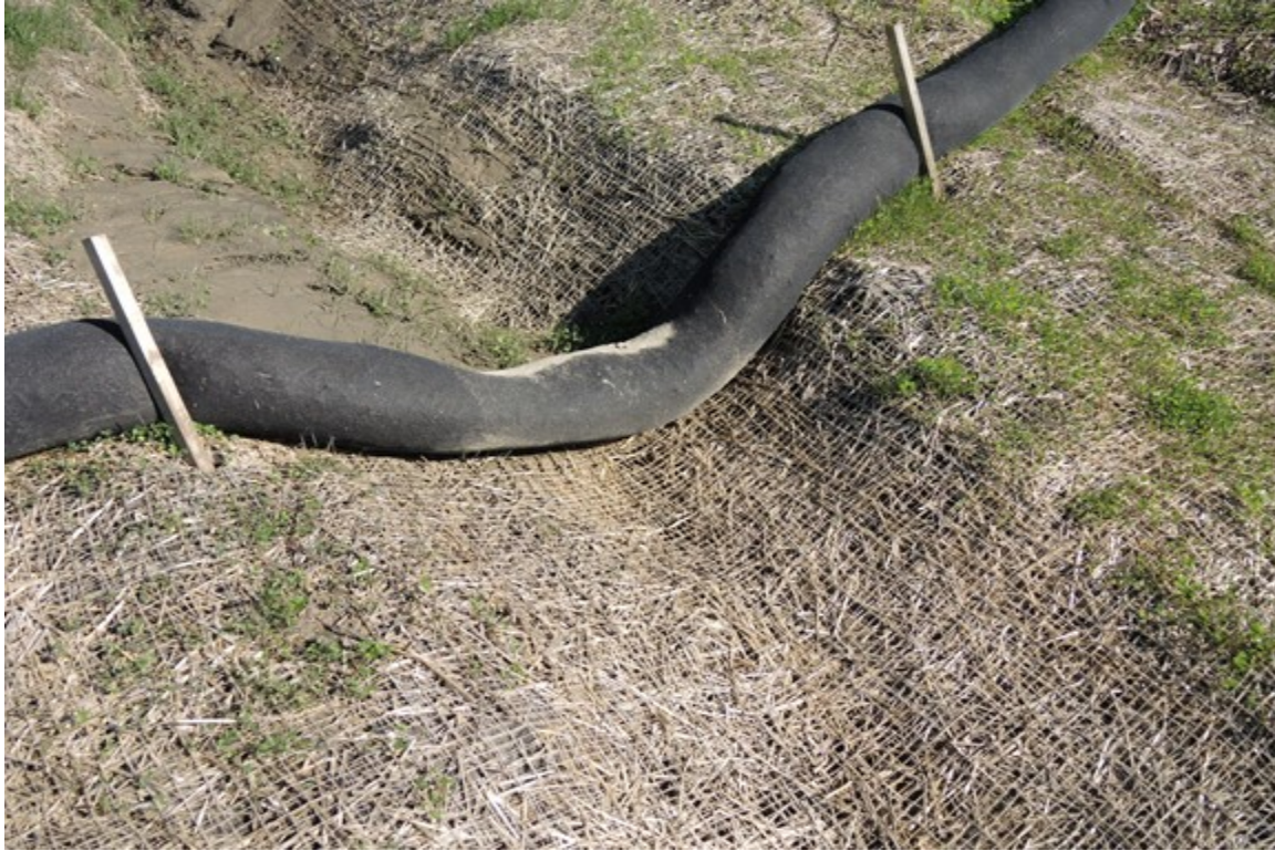
Figure 32 Product chosen could not handle the flow at this location. Another sediment control log that could withstand higher flows would be a more appropriate choice.
