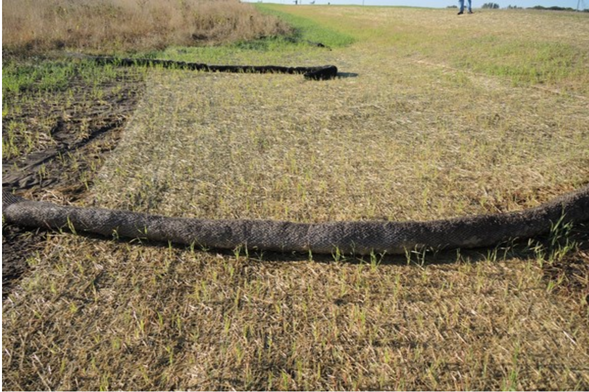
Figure 31 Product installation error allowing flow to go around the product.
