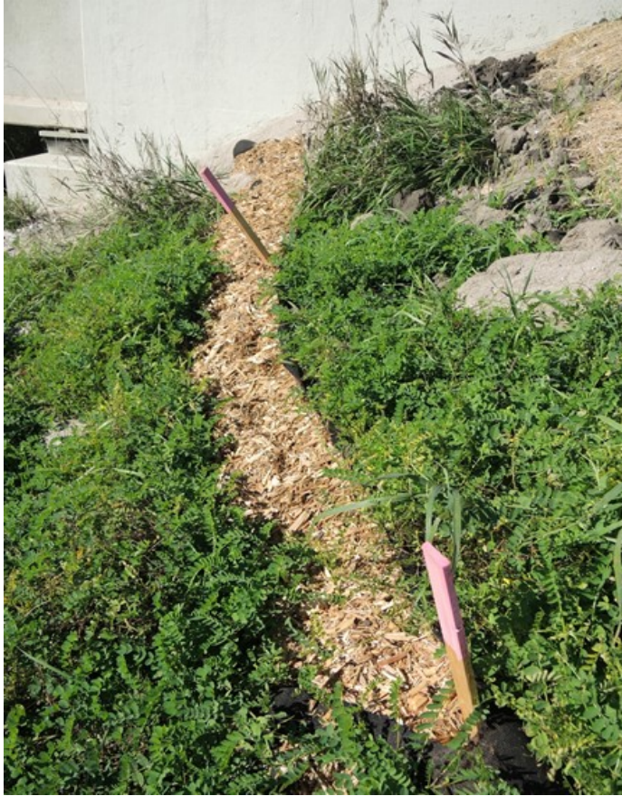
Figure 33 Product required maintenance prior to its current state. Replacement at the time of the photo is required to continue controlling erosion at the site.
