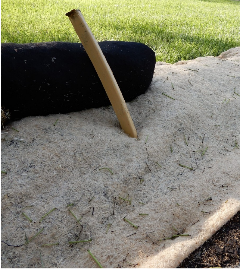
Figure 37 A partial installation of a wood compost sediment control log along a perimeter. The foundational blanket extending past the log will offer some protection in case of overtopping.
