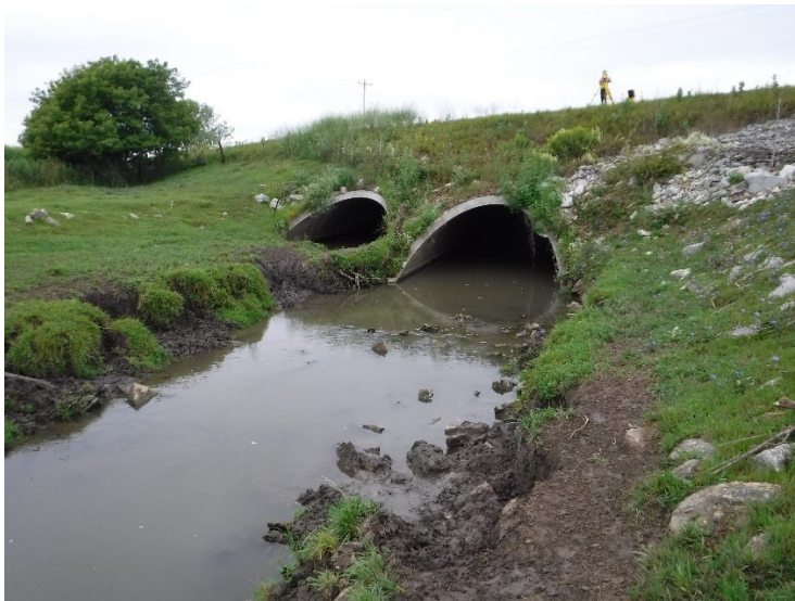
Figure 40. Culvert exit. August 14, 2019. Barrel 2 had significant sedimentation.
