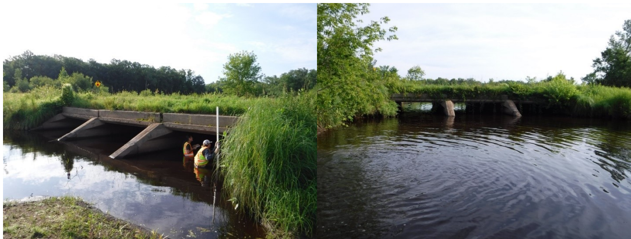
Figure 38. Culvert entrance (left) and exit (right). August 2, 2019. No barrels were embedded or offset.
