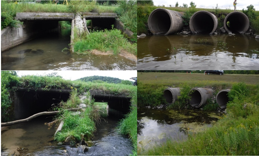
Figure 6. Photo documentation of culvert inlets (top) and outlets (bottom) from the Root River (left) and Red Lake River (right).
