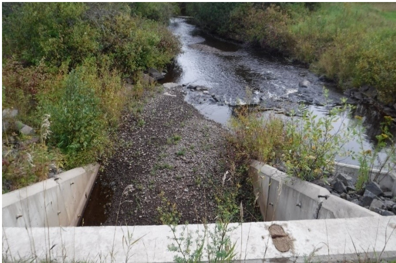
Figure 33. Grade control was provided by a weir downstream.
