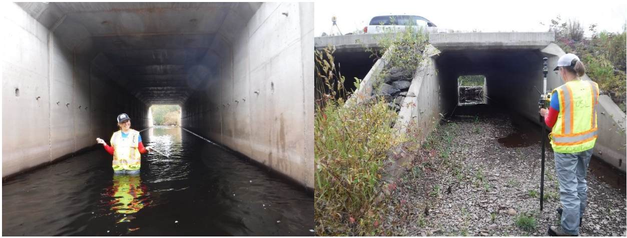
Figure 32. Photos of embedded barrel (left; barrel 2) and offset barrel (right; barrel 1). September 27, 2019.
