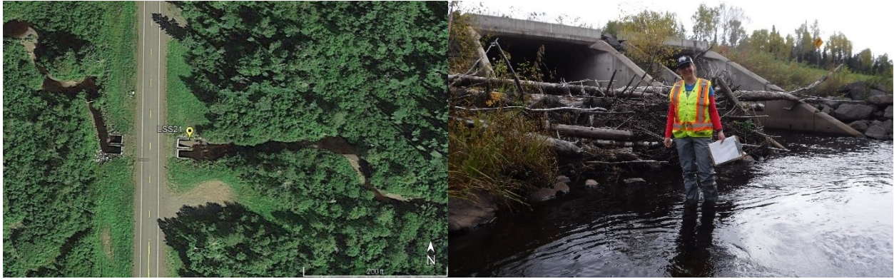
Figure 31. Aerial image of LSS21 showing skewed culvert entrance. Flow is from left to right (left). Woody debris caught on culvert entrance (right).
