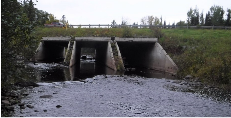
Figure 36. Grade control was provided by a weir downstream.
