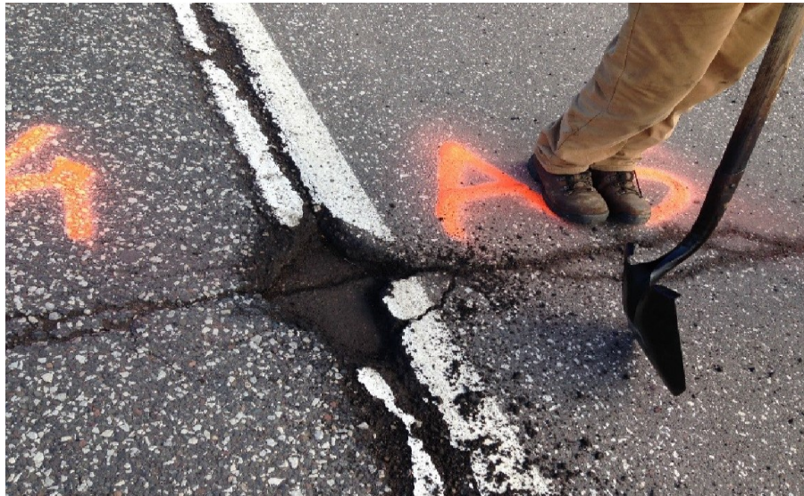
Figure A.10 Photograph of a Pothole (Dailey et al., 2017)
