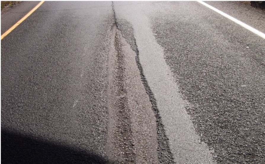
Figure A.16 Raveling in Asphalt Pavement (MnDOT, 2011)
