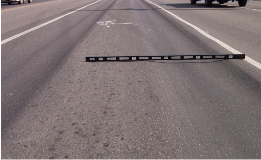
Figure A.15 Rutting, 0.50 inches Deep or Greater (MnDOT, 2011)
