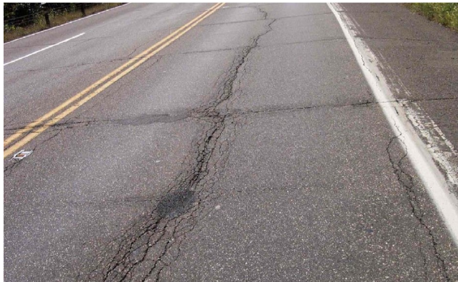
Figure A.6 High Severity Longitudinal Crack (MnDOT, 2011)
