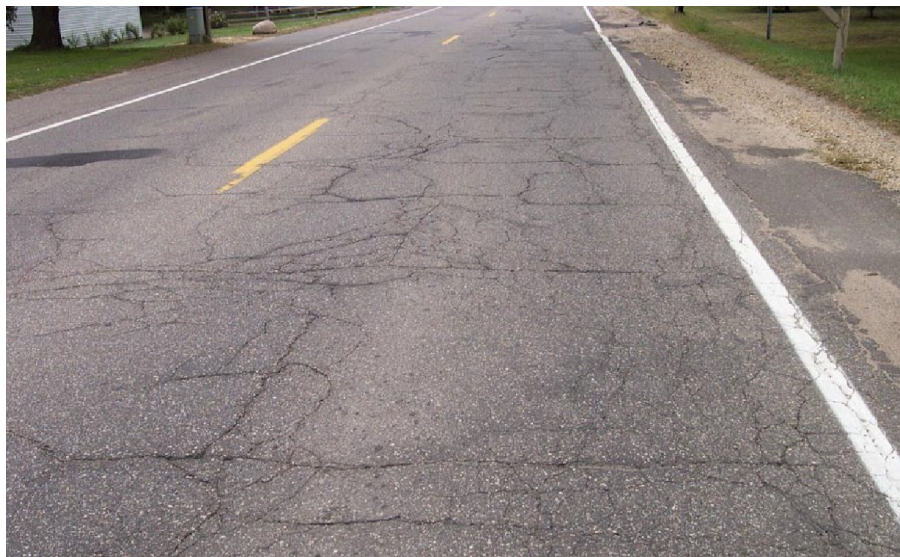
Figure A.12 High Severity Multiple Cracking (MnDOT, 2011)
