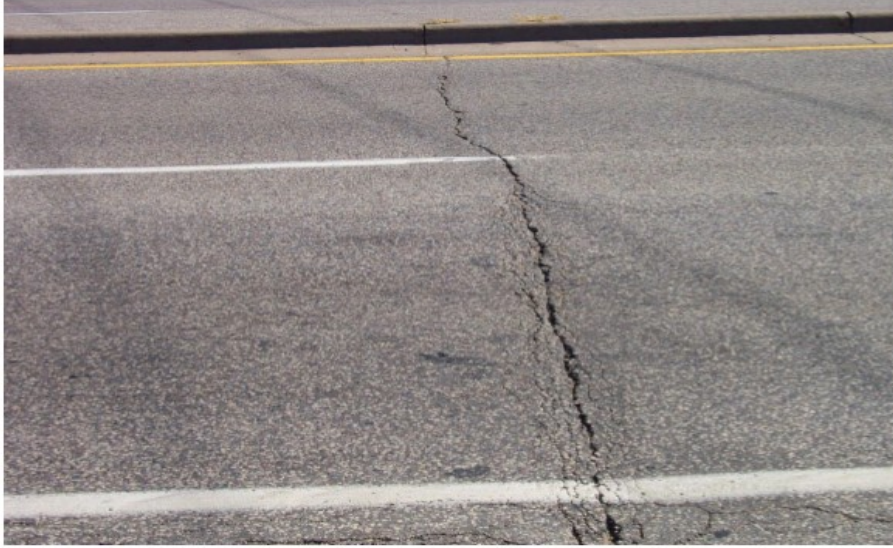
Figure A.3 High Severity Transverse Crack (MnDOT, 2011)
