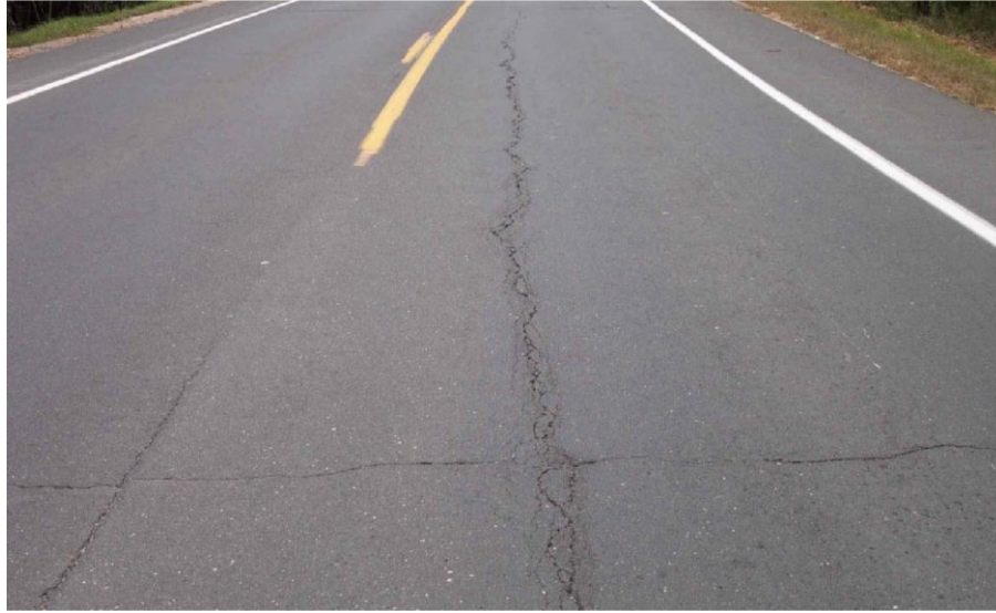
Figure A.5 Medium Severity Longitudinal Crack (MnDOT, 2011)
