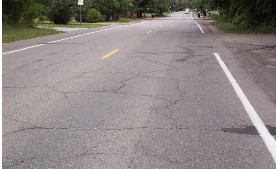
Figure A.11 Medium Severity Multiple Cracking (MnDOT, 2011)
