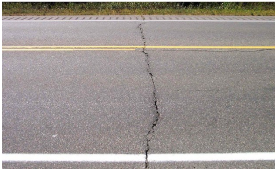
Figure A.2 Medium Severity Transverse Crack (MnDOT, 2011)
