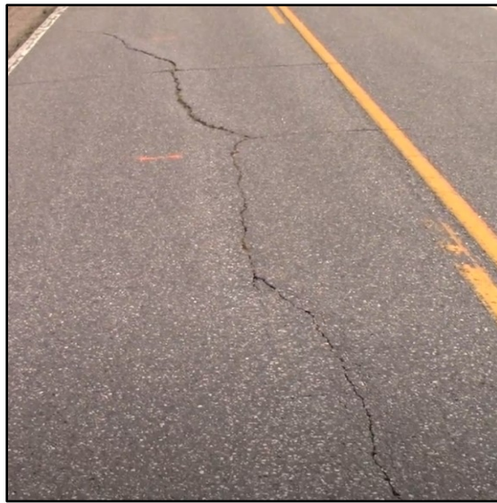
Figure 4-14 Medium severity longitudinal cracking in Koochiching County
