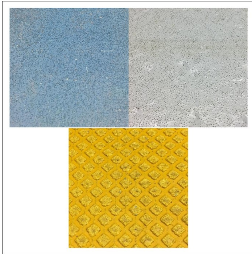
Figure 2.4 Slab surface markings for a) paint with beads, b) thermoplastic with beads, and c) cold-applied preformed tape (Nassiri, 2018)
