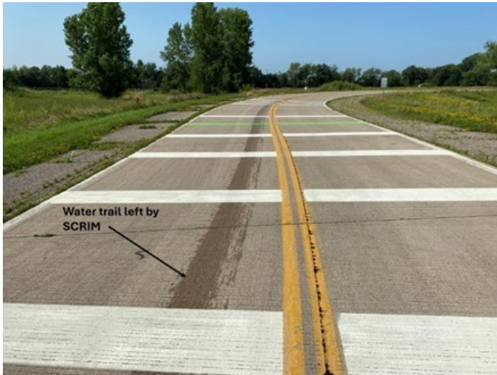
Figure 5.8 Water trail left by SCRIM on Cell 46 pavement
