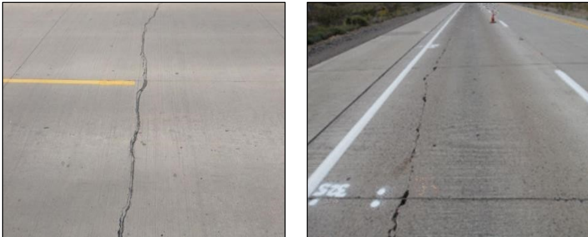
Figure 2.1 Transverse crack (left) and Longitudinal crack (right) (Harrington et al., 2018).
