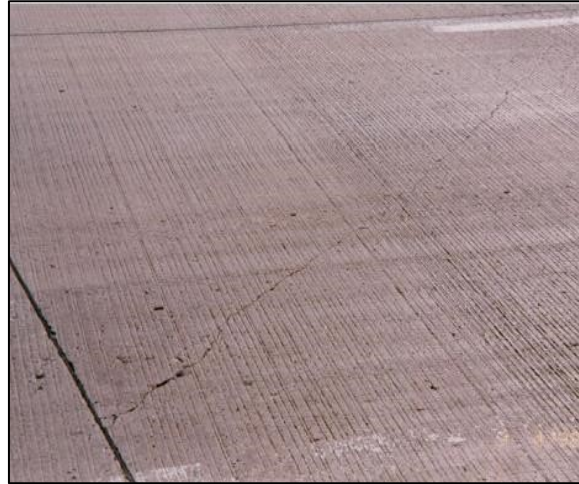
Figure 2.2 Diagonal cracking (Harrington et al., 2018).
