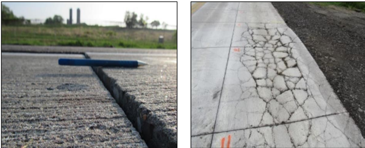
Figure 2.3 Joint Faulting in thin pavement (left) and slab shattering in ultra-thin fiber reinforced pavement(right) (Barman et al., 2021).
